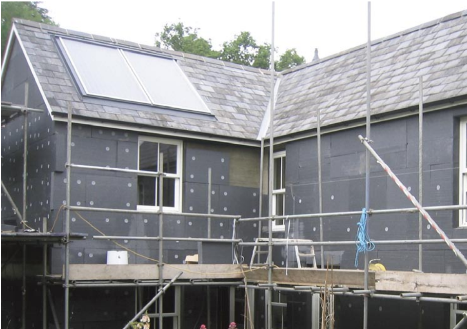
This extensive retrofit included external wall insulation (EWI) but also new roof, new windows, and an extension. Solar thermal panels were also installed. The clients wanted to save energy and make their home nicer to live in. Gas bills have fallen by roughly 50%, the house is much warmer, and it no longer suffers from condensation and mould growth. Photo: Alan Clarke
