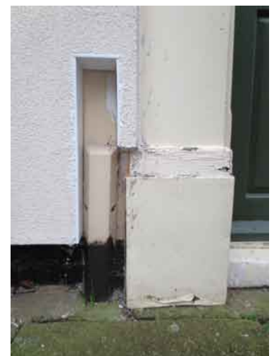
The installers did not have a good strategy for dealing with this service entry, and there is a very large thermal bridge at the porch. Courtesy of NDM Heath Ltd
