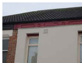
Leaving the decorative band at the top of this wall exposed has created a large thermal bridge, and may increase the risk of rain penetration. Courtesy NDM Heath Ltd
